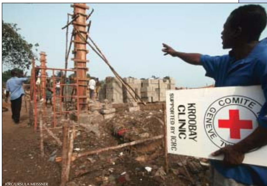
Healthy Recovery. An International Committee Red Cross official directs the construction of the new Kroobay clinic in Freetown, Sierra Leone.
