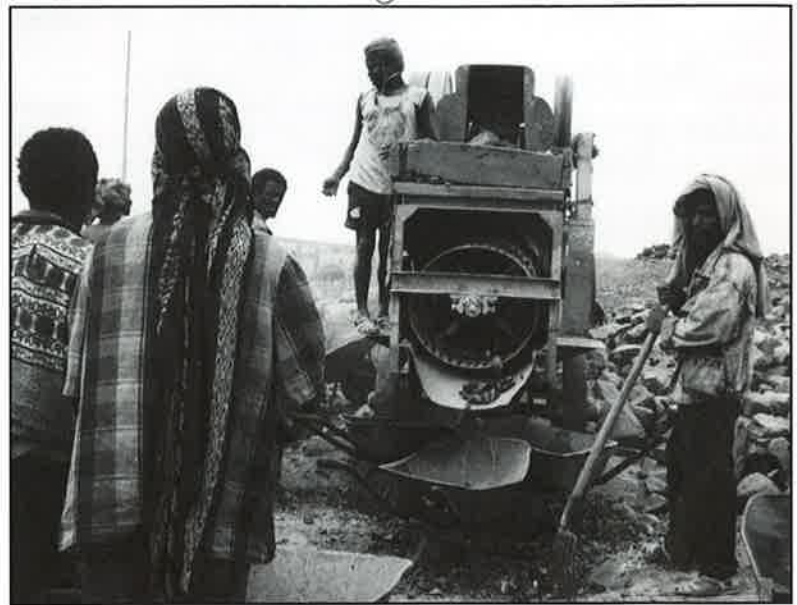
Reviving Old Connections. Rebuilding the old Italian narrow-gauge railway that connects the sea to the inland is vital to Eritrea's economic development.
