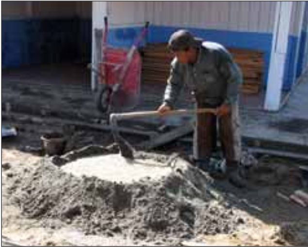
A worker prepares concrete at the site of an American-funded market project in Ronga Ronga, Indonesia. (photo by Kristin McHugh/The Stanley Foundation)
